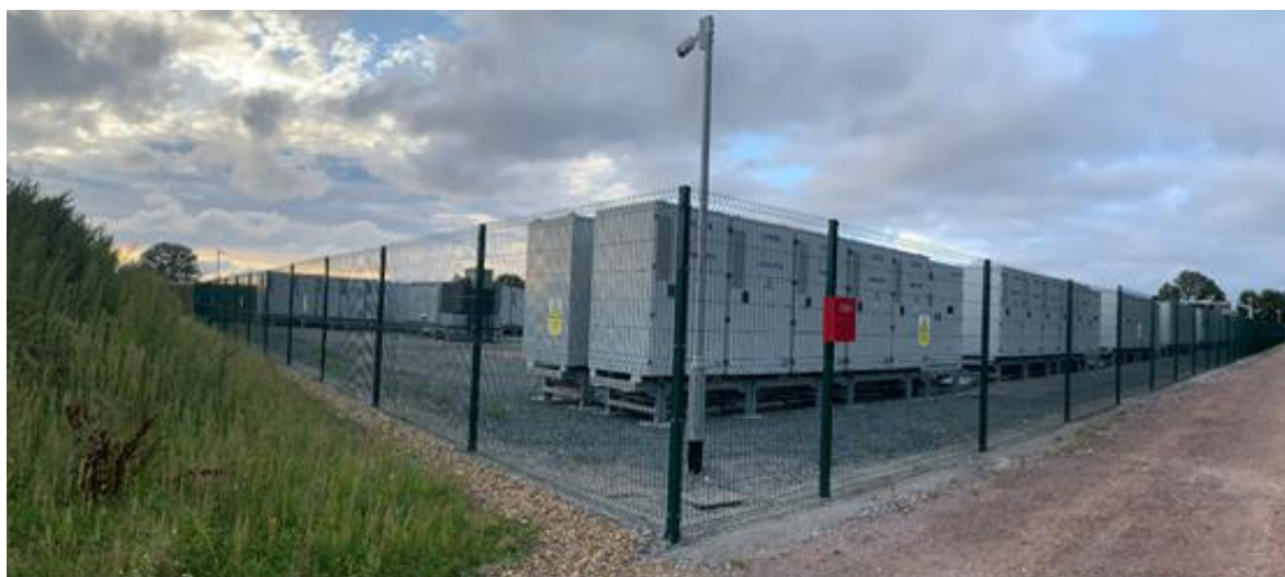
Figure 15-19: Example of a BESS
