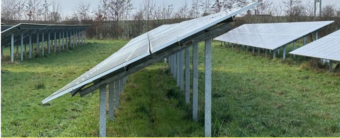
Figure 15– 22 : Panels Array Showing Gaps Between Panels
