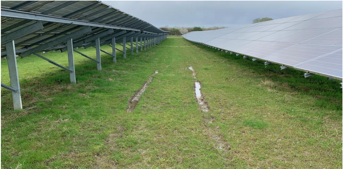
Figure 15–21: Example of Minor Ruts Caused by Vehicles
